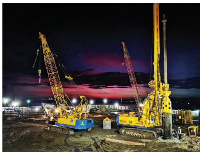
TOP (LEFT AND RIGHT): Bauer BG 40 rig carried out drilling work for a geothermal power plant on the island of Leyte.
