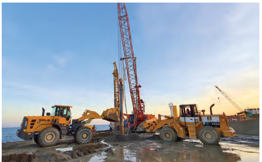
TOP: Since August 2019, Bauer has been involved in the expansion of the highway between the cities of Sucat and Alabang in southern Metro Manila.
