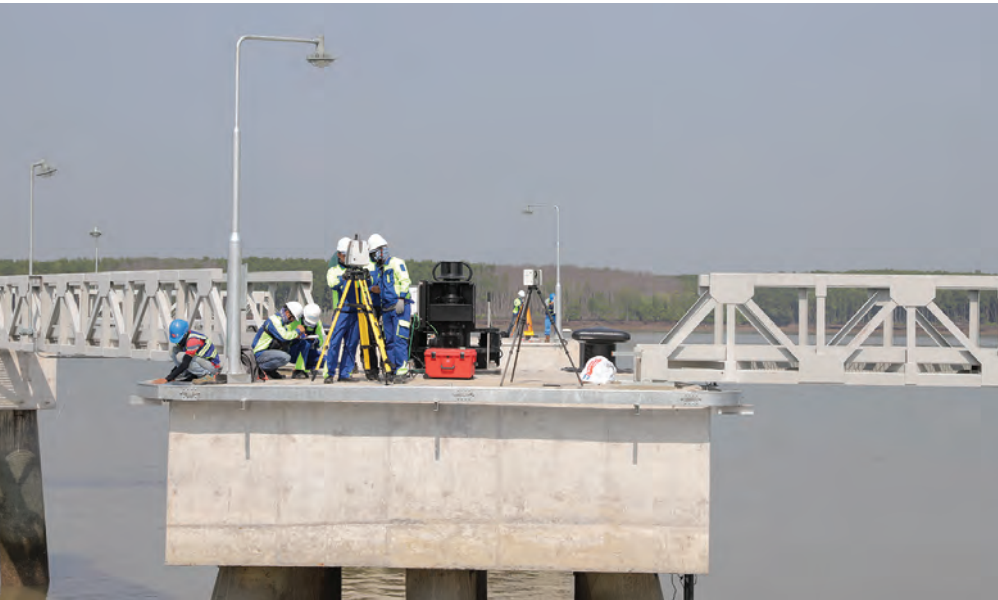
LEFT: Portcoast carried out the project with the help of Leica Geosystems' products. Among them was the ScanStation P50 laser scanner (pictured), which was used to capture the data on top of the bridge.
