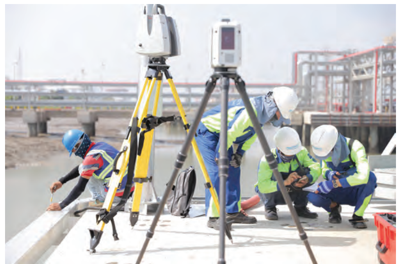
TOP: The construction of Hyosung Vina Chemicals Port in the Ba Ria-Vung Tau province, southern Vietnam, began in 2018 and was completed in March 2020.
