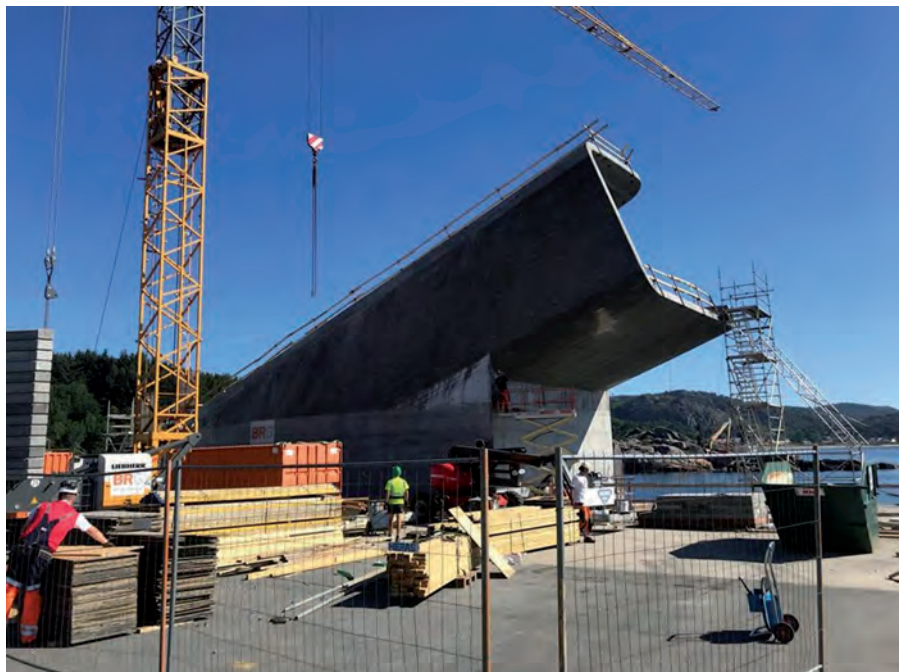
TOP: Located 5 m below sea level, the Under restaurant is made from precast modules and is anchored to a block of concrete.
